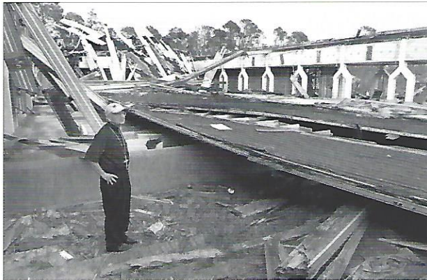
ARCHBISHOP Alfred C. Hughes examines the collapsed roof of Our Lady of Lourdes Church in Slidell that was caved in by the 145 mph winds of Hurricane Katrina Aug. 29. Archbishop Hughes toured many of the damaged churches and schools in St. Tammany Parish on Sept. 17 and celebrated Vigil Mass in the Our Lady of Lourdes cafeteria. The archdiocese is conducting a structural and environmental assessment of its churches, schools and other properties in the most affected areas. St. Bernard and lower Plaquemines civil parishes and parts of Orleans Parish. An inconclusive archeological analysis indicates flood damage to archeological facilities - not including wind damage - could amount to $84 million. About 70 of the archdiocese's 143 parishes are up and running. (Photos by Patrick J. Neenan)
